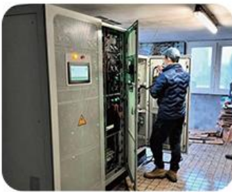
Industrial energy storage
