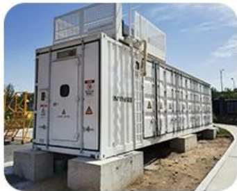
Communication base station energy storage
