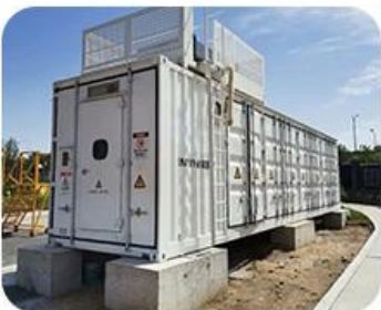
Communication base station energy storage
