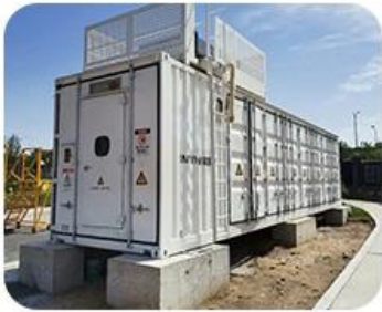
Communication base station energy storage
