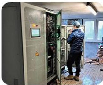
Industrial energy storage
