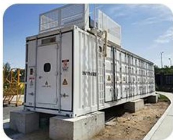
Communication base station energy storage
