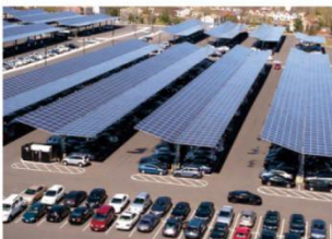
Commercial car park
